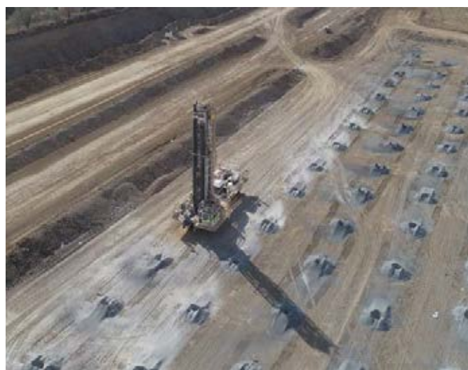
Picture 2: Remotely operated, semi-autonomous drill is successfully operating at our Dawson mine.
