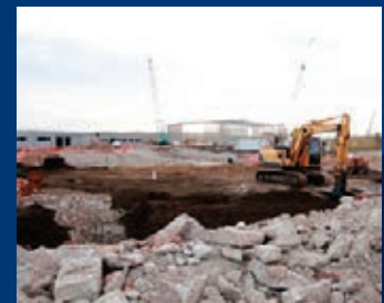
CAVAL RIDGE GENERAL SERVICES MORANBAH, QLD BECHTEL AUSTRALIA PTY LTD
